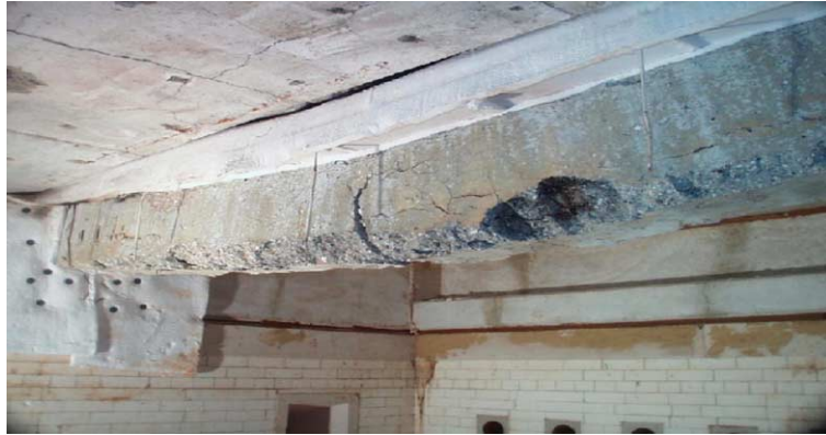
Fig. 8. Rupture at the mid-span of the concrete in beam 1 after fire.
