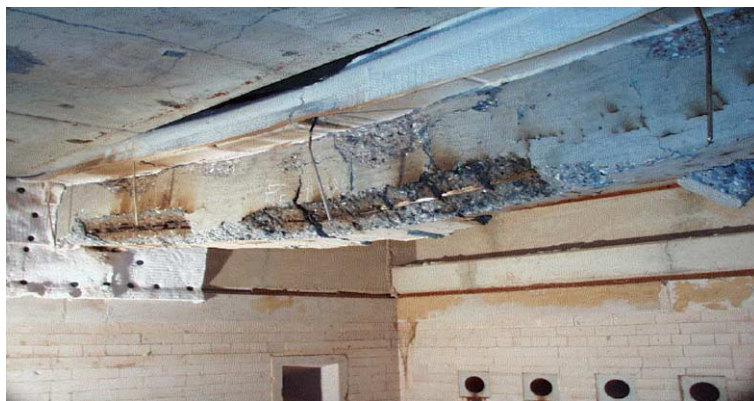
Fig. 9. Failure of beam 2 after fire test inside the furnace shows some flexural cracks and rupture in the main reinforcement.
